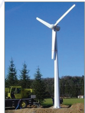
50 kW wind turbine
